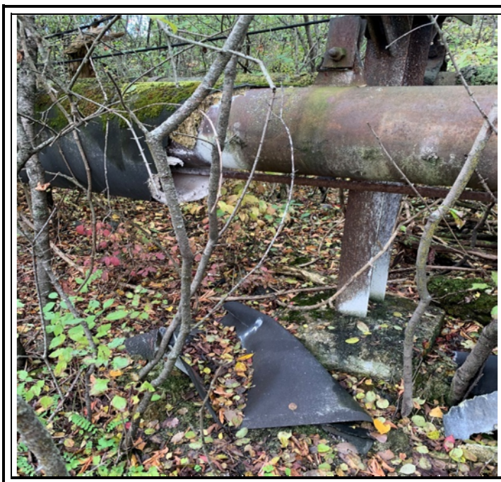
Photo 8 - Typical pipe insulation debris between Points B and D
