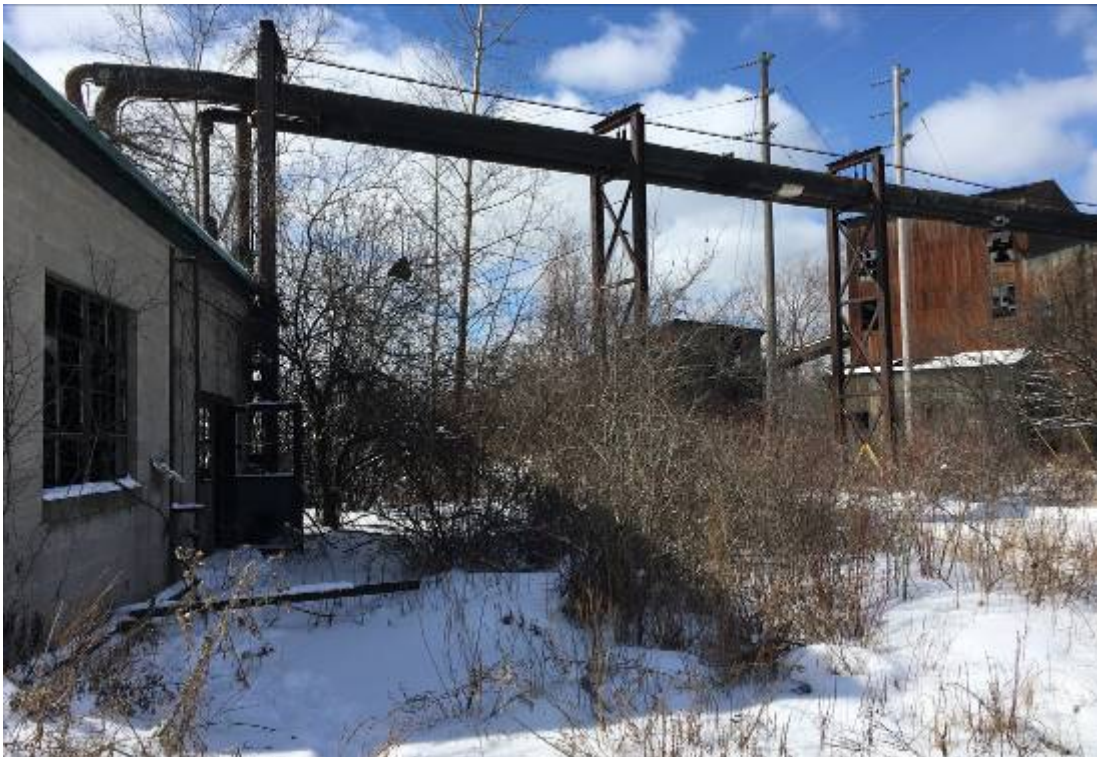
Exterior of building (at left) with ACM piping on overhead rack towards conveyor area
