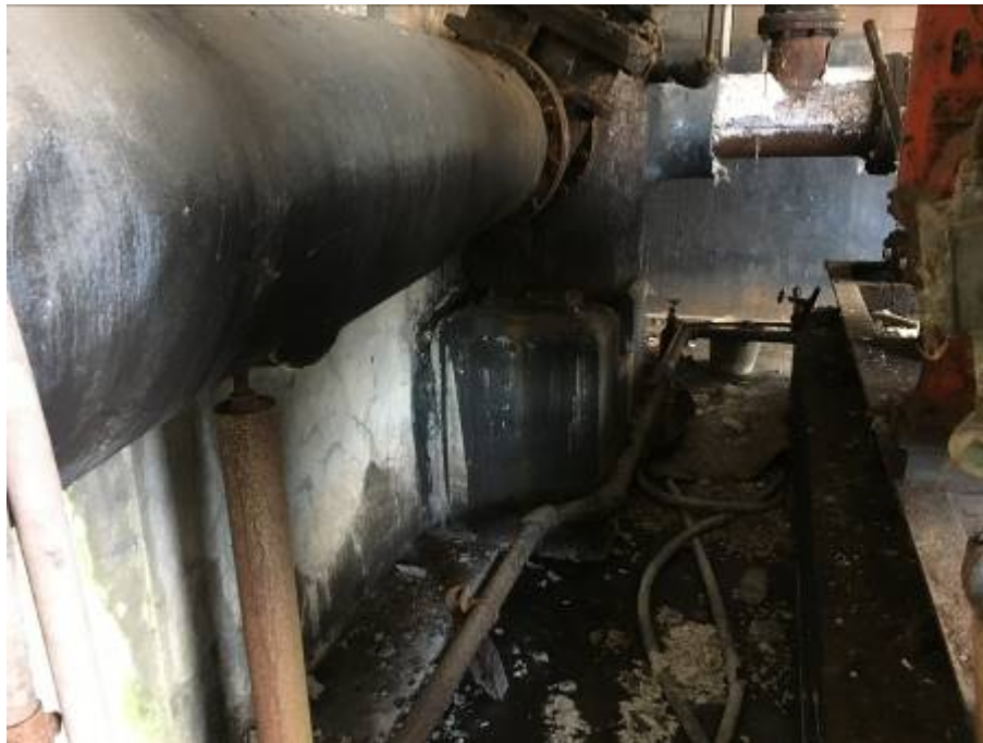
ACM pipe insulation debris on surfaces in many areas
