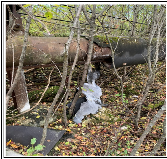
Photo 6 – Typical pipe insulation debris between Points B and D
