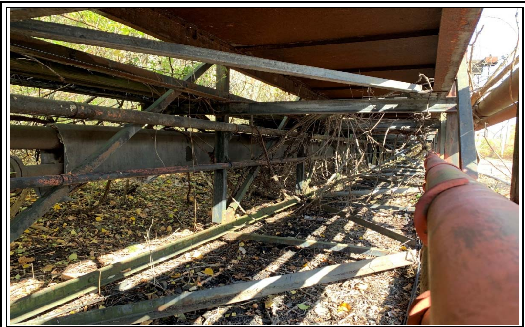
Photo 2 – Typical pipe insulation with overhead protection between Points A and B
