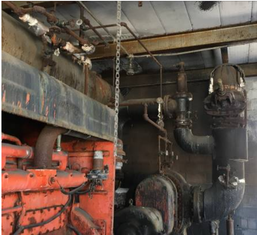
ACM pipe and fitting insulation in poor condition near ceiling and at pump
