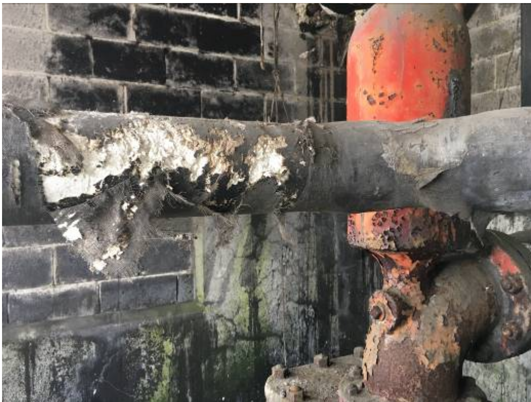
Black cloth pipe wrap over white pipe and fitting insulation
