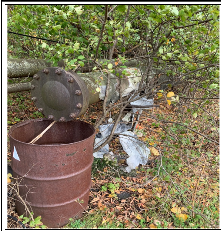
Photo 7 - Typical pipe insulation debris between Points B and D
