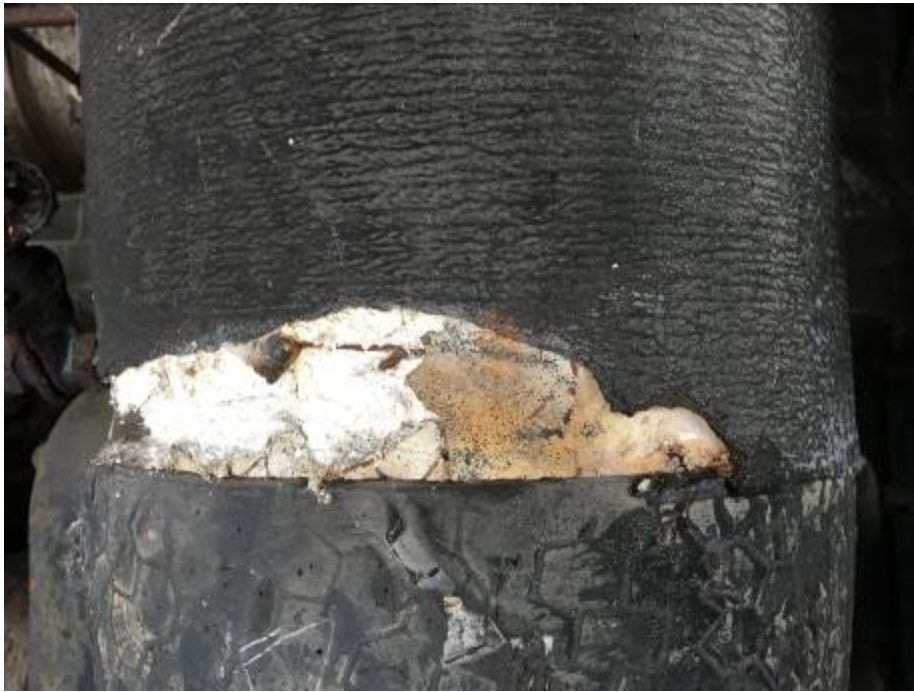
Black pipe wrap with wire (lower pipe) and tar-paper-like wrap on upper pipe
