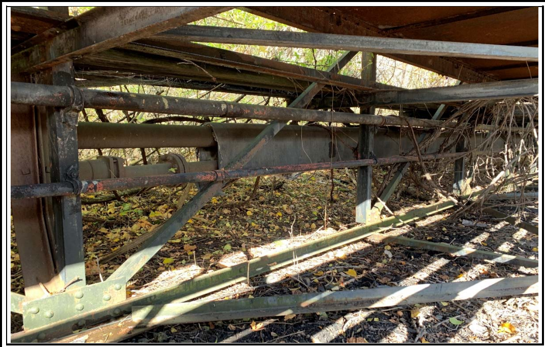
Photo 1 – Typical pipe insulation with overhead protection between Points A and B
